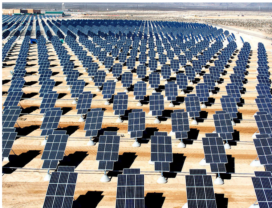
Figure 3 - Portion of the Nellis AFB 14 MW PV system (distribution-connected).
