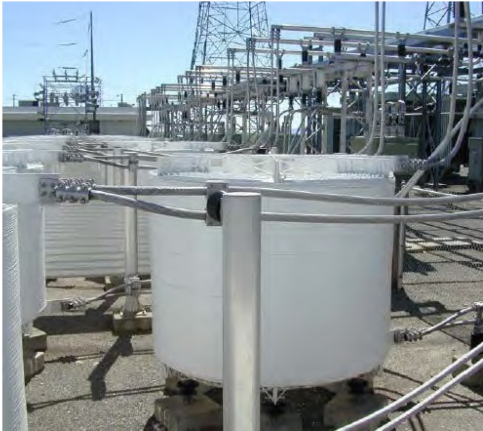
Figure 5.11: Low-Voltage Tertiary Reactor (13.8kV)
