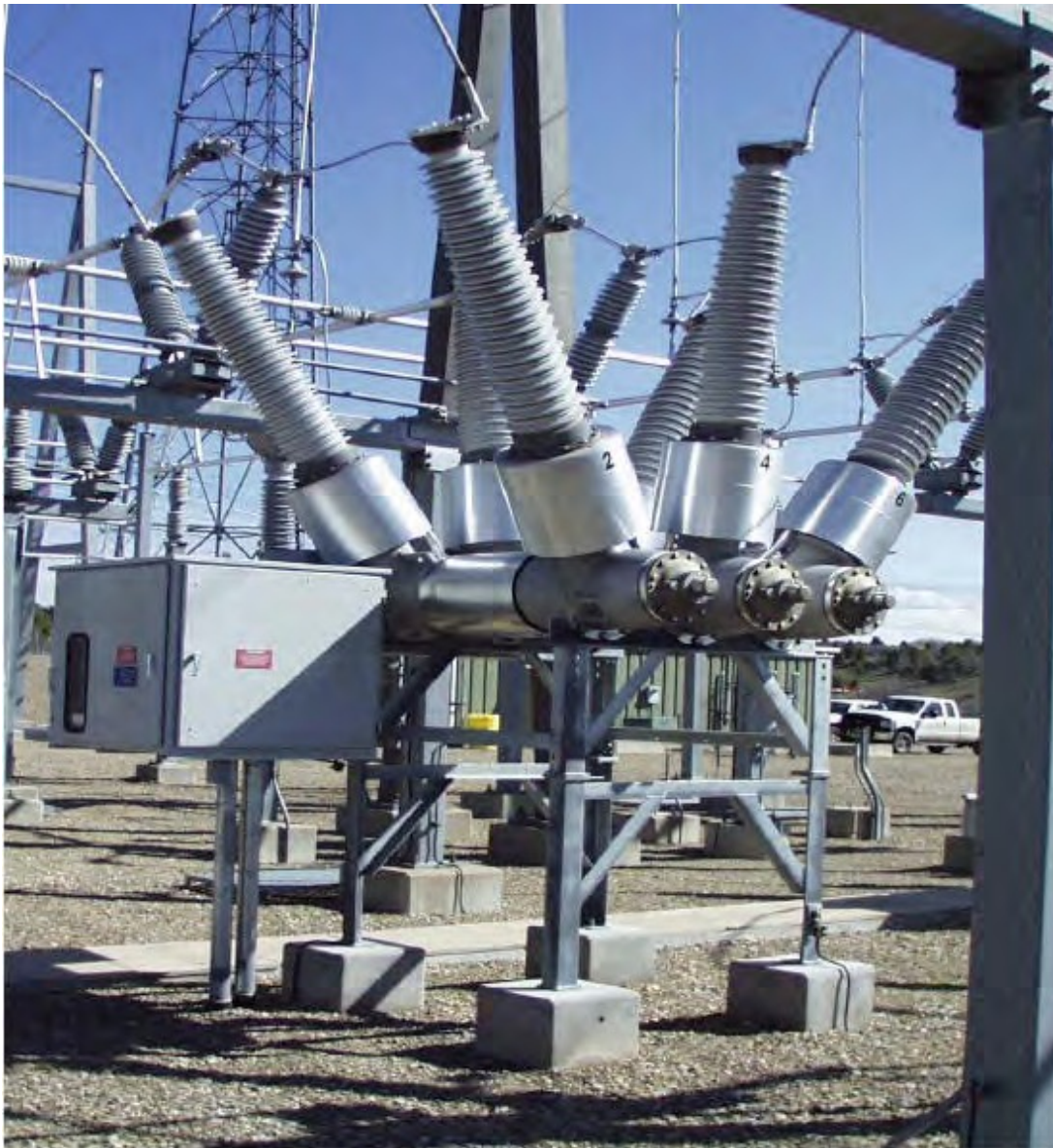
Figure 5.6: 115kV Gas Puffer Circuit Breaker
