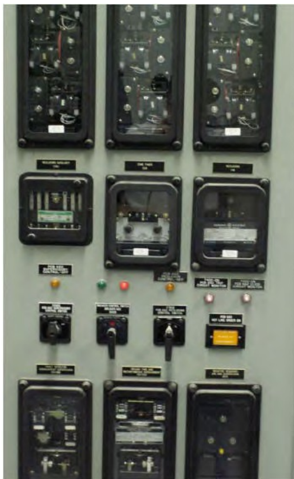
Figure 5.17: Transmission Line Relay Panel
